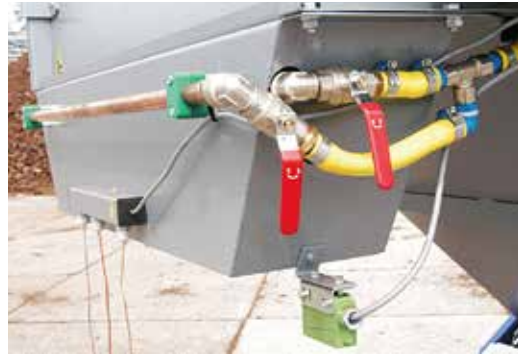
Water dosing system
